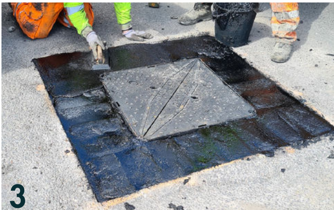
3 Additional mastic asphalt is applied to fill the voids and create a monolithic structure. The surface is hand levelled.
