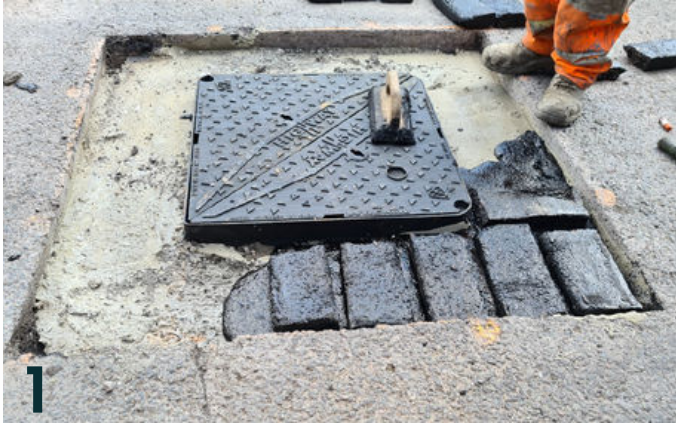
1 Break out and replace the existing ironwork and bed in rapid-set mortar. Infill with hot polymer-modified mastic asphalt.
