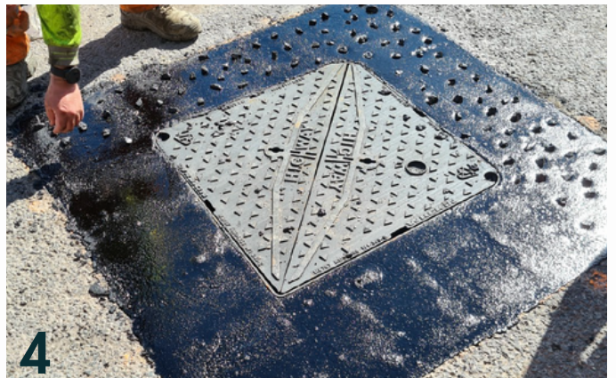
4 Pre-coated asphalt chippings are embedded in the surface of the mastic-asphalt creating a positive surface texture and skid resistance.
