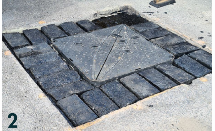
2 Cold mono-polymer bricks are laid to cool the hot mastic asphalt and provide structural ability.
